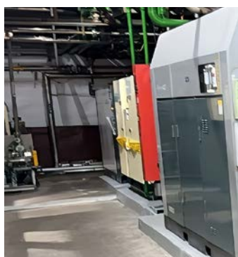
Compressed air system in Zone 07
