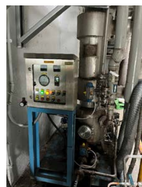
▲ Vacuum pump and water recovery system
