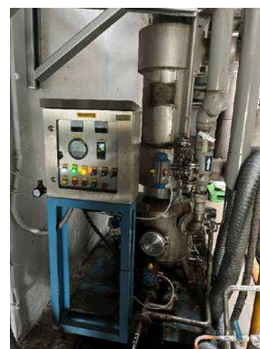
▲ Vacuum pump and water recovery system
