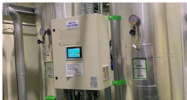
▲ 07 Area – High consumption air dryers
