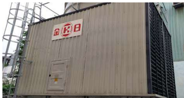
▲ 300RT ice water machine and cooling towers in the Research Building upgraded.
